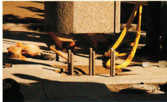
After careful fabrication, each pillar was carefully installed on its onsite support box. Alignment was critical, both for the support of the columns and to provide a steady flow to the water feature located at the top of each column. (Photos courtesy Jensen Corporation Landscape Contractors).
