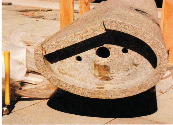
Creating the elliptical pillars was handled by Granicor at its Alma, Que., plant. Each was made in three pieces. Because of the shape, each was cut and ground individually. In assembling the pieces, the company also had to meet California's stringent seismic regulations. (Photo courtesy Jensen Corporation Landscape Contractors).
