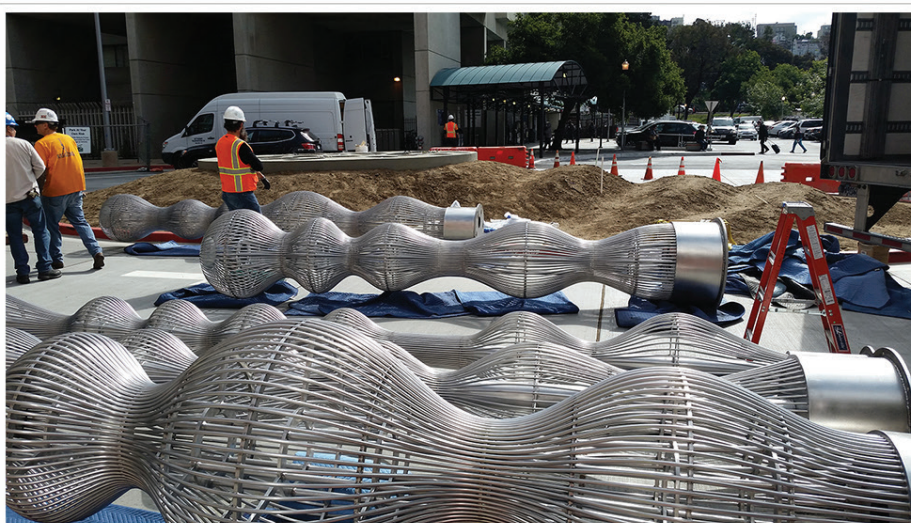
As seen during the installation of the artwork, the earthwork's wave like berms form a shape similar to the profile of the sculpture. (Photo: Cliff Garten Studio)
